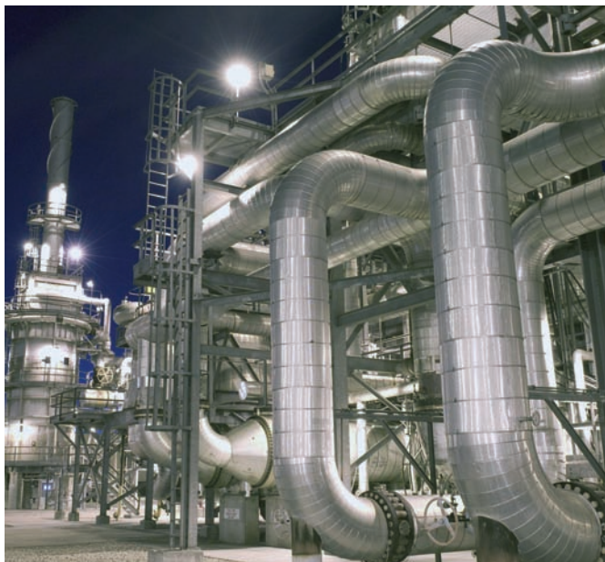
The Great Plains Synfuels Plant in North Dakota, U.S., has been producing natural gas from coal for over 25 years.
