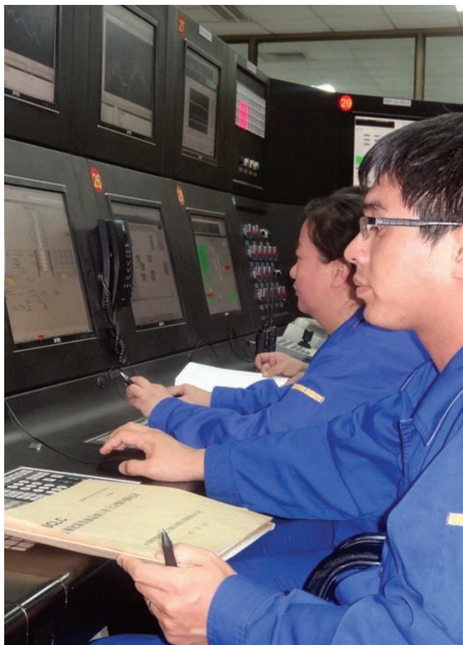
Researchers at the National Institute of Clean and Low-Carbon Energy monitor operations of an ICTL project.
