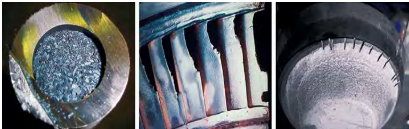
FIGURE 1. Oxide deposits on boiler tubes (left) and solid particle erosion on turbine blades (center) and bypass valve plug (right)
