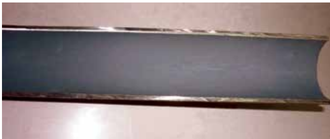
FIGURE 2. Pipe from the second reheater tube after 30 months of operation
