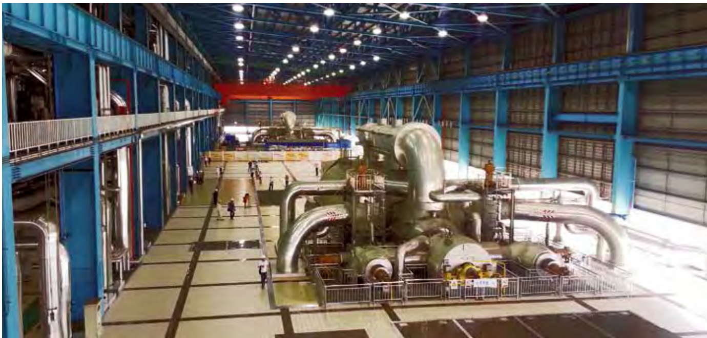
Steam turbines at the ultra-supercritical Waigaoqiao No. 3 (Shanghai) (photo courtesy of IEA CCC)
