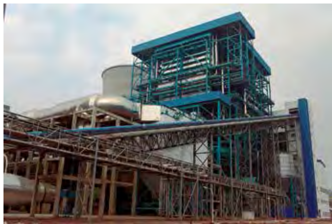
The 600-MW SC CFB boiler
