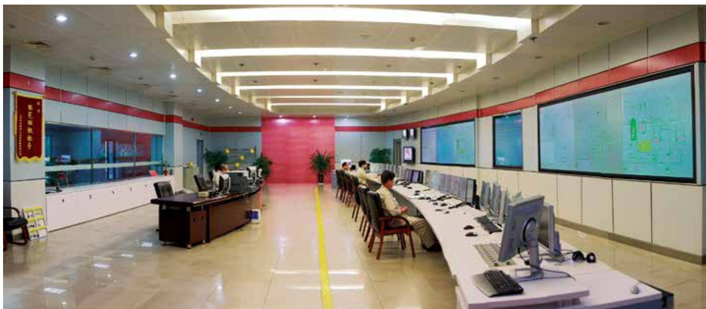
Operators monitor plant operation at Waigaoqiao No. 3.
