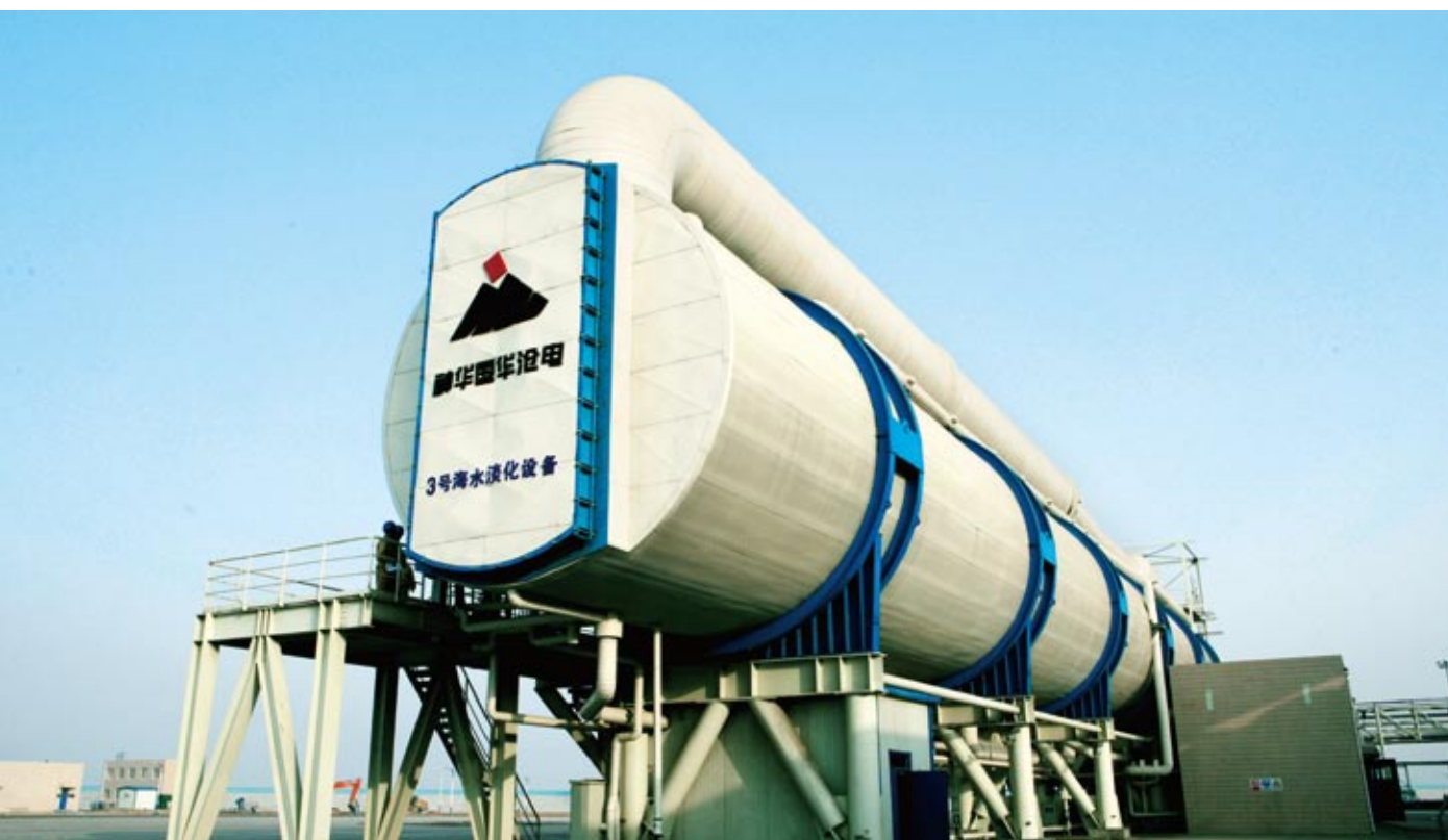
神华国华沧东电厂海水淡化装置 Sea water desalination facility of Shenhua Guohua Cangdong Power Plant
