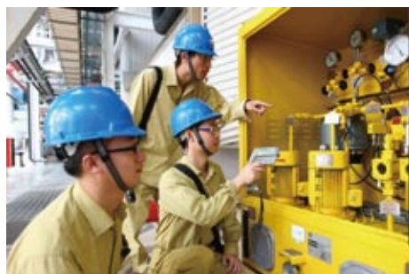
设备维护点检人员对风机油站进行巡检 Maintenance staff inspecting oil station of the wind turbine
